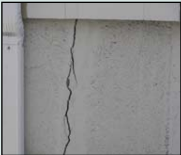
A cracked foundation can lead to serious problems. We can Help.
